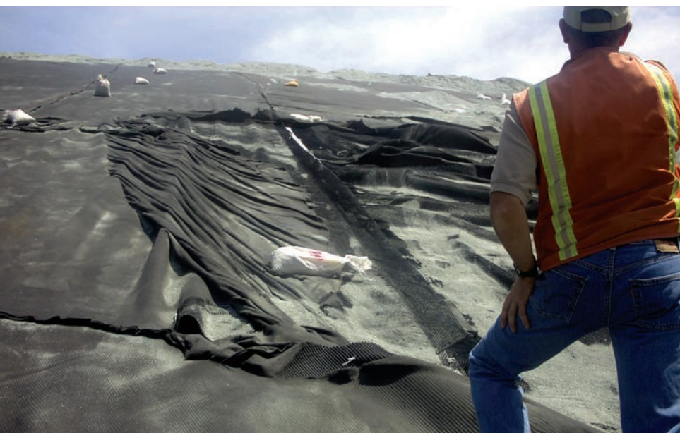
FIGURE 4 Geocomposite adhesion failure in the field after attempted soil covering
