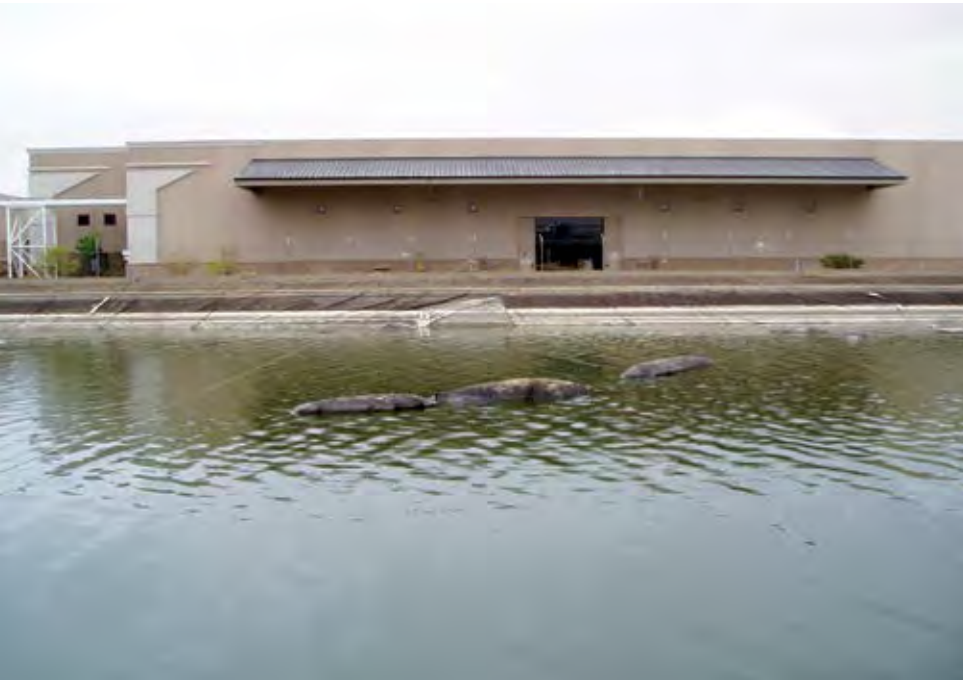
Figure 2 Bubbles in a wastewater pond caused by gases generated from wastewater that leaked below the geomembrane
