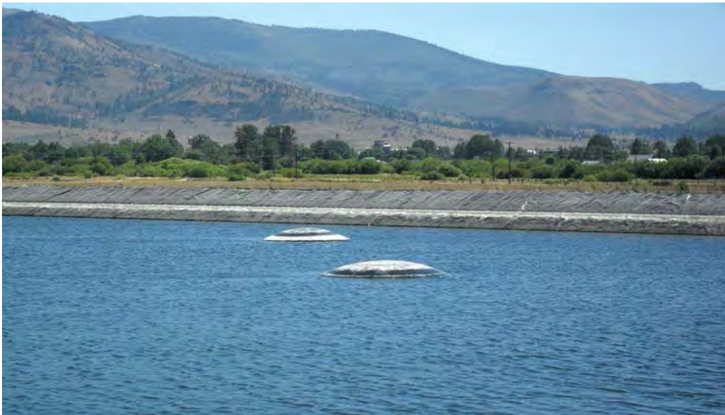
Figure 5 Bubbles in a pond with 1.5-mm (60-mil) geomembrane on the verge of bursting (another one did burst two days before this)
