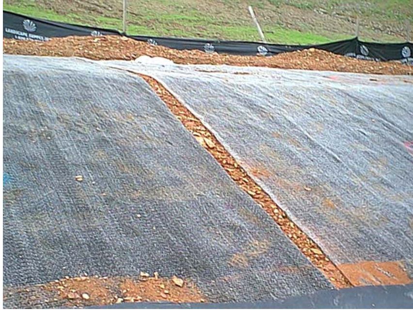
Figure 1. Photograph showing gap in GCL panels after removal of geomembrane.
