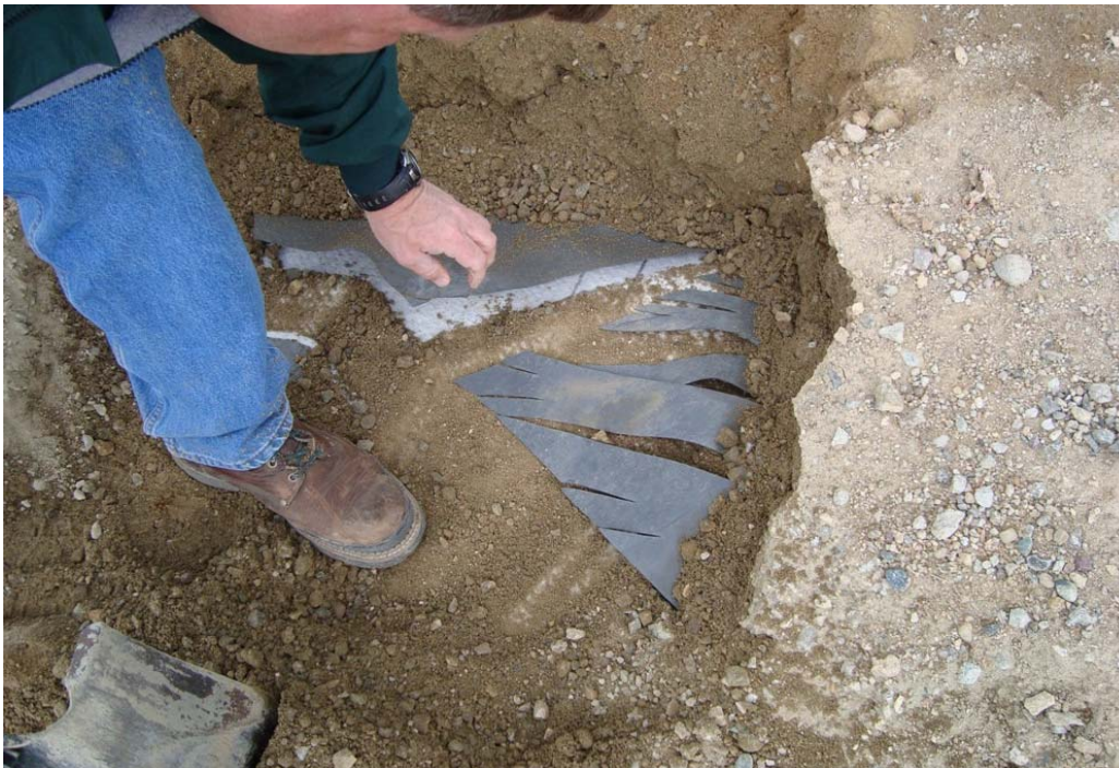
Figure 5. Standing on exposed GCL (obscured with sandy gravel cover) and lifting edge of torn PVC. Clean white GCL can be seen been raised edge of torn PVC. Condensation water was noted on bottom side of PVC.
