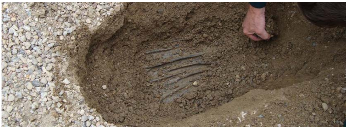
Figure 3. Bunched-up wrinkles in PVC at toe of 4:1 slope.
