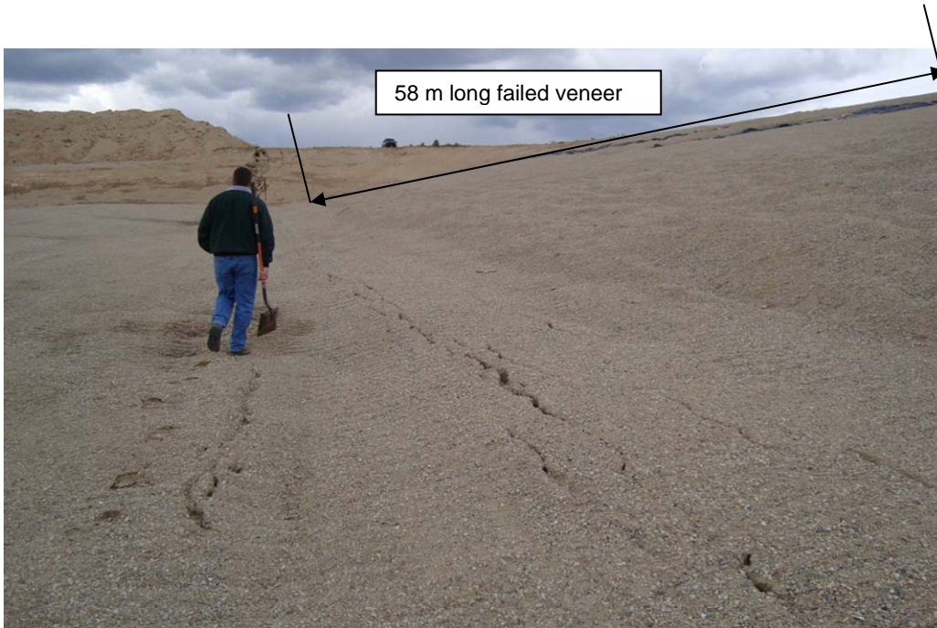
Figure 4. Deformed and cracked cover soils near toe of slope.
