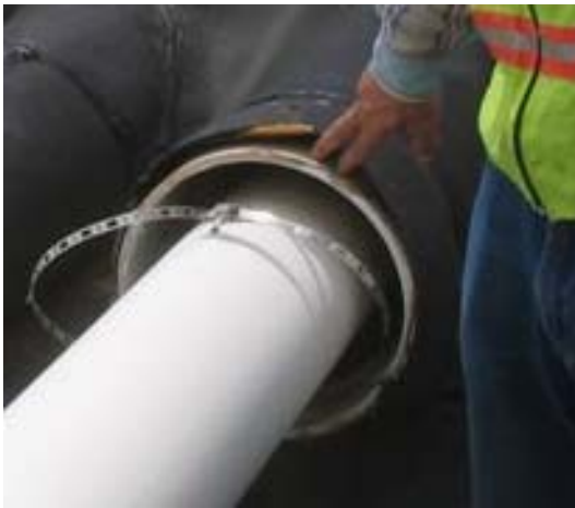
(c) Thin band clamp that has loosened and come off.
