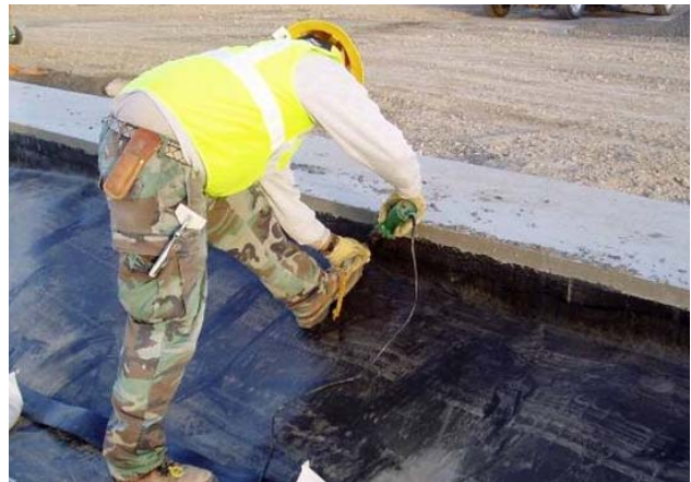
(b) Heat tacking geomembrane to embedment strip after the concrete was placed and forms were removed.
