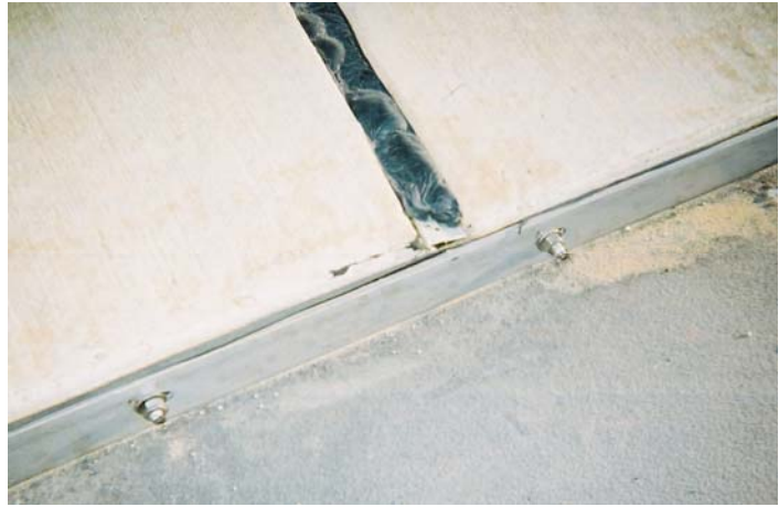
(b) Bad concrete joint will defeat batten when submerged.
