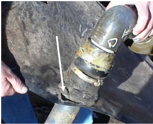
(a) Failed pipe boot at skirt-to-sleeve weld.
