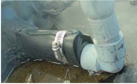
(a) Classic example of poorly constructed boot that violates all good construction principles.
