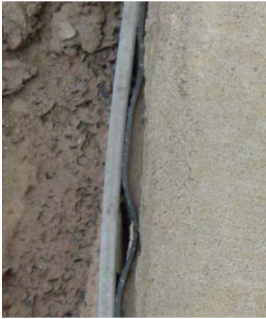
(a) Wavy substrate will cause leaks.
